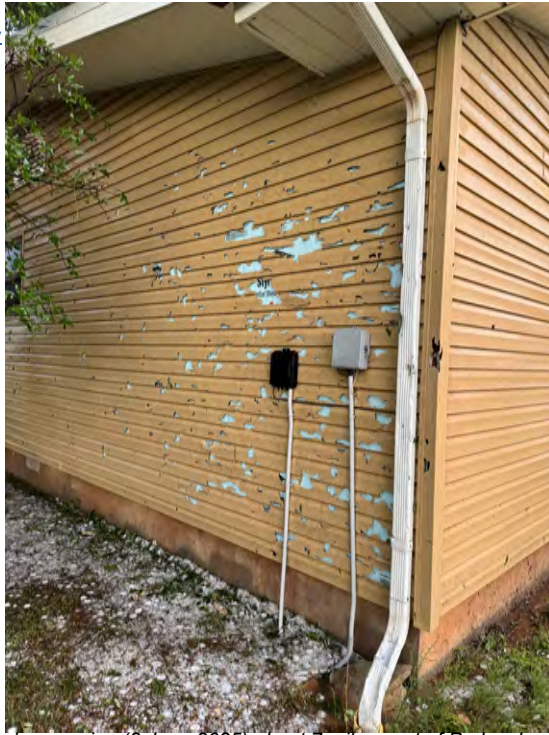
Pictures of hail and wind-driven hail damage incurred on Sunday evening (8 June 2025) about 7 miles east of Paducah. The pictures are courtesy of Dana Wright.
